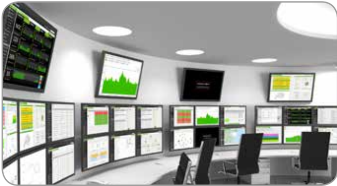
SCADA/Energy Management/Distribution Management Systems
